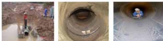
Figure 5: Accumulation of mud, sand, and plastic particles inside the valve cavity.
