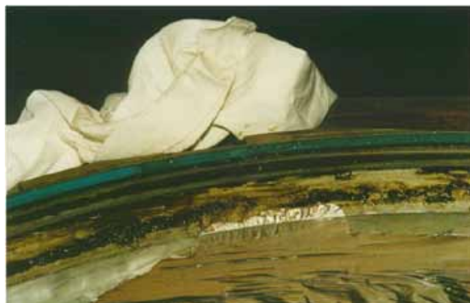
Figure 6: Melting of the soft seat insert during preheating.
