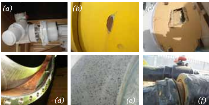
Figure 2: Example of identified damages during valve receiving inspection: (a) actuator damage; (b) damage to a valve's external coating; (c) flange cover damage; (d) uniform corrosion in the valve cavity due to improper drainage procedure; (e) pitting corrosion in a ball service; and (f) valve riser damage.
