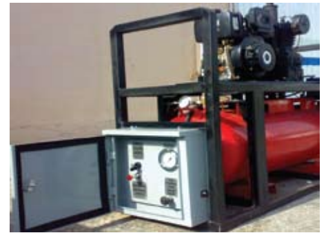
'Figure 2: The Air feed Skid'
