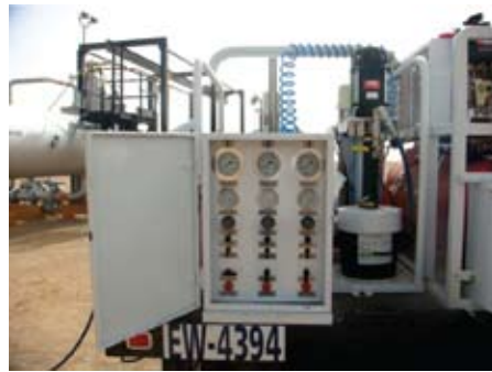
'Figure 1: Pump Control Cabinet'
